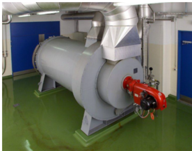
Figure 4: A oil fired hot air generator.
