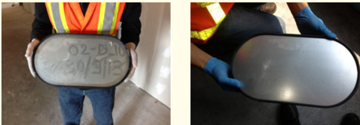
Figure 3: Dust on internal surface of air duct access door.
